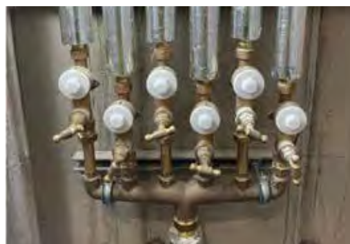
Stopcock in communal cupboard
