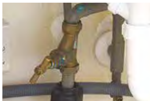
Stopcock inside utility cupboard
