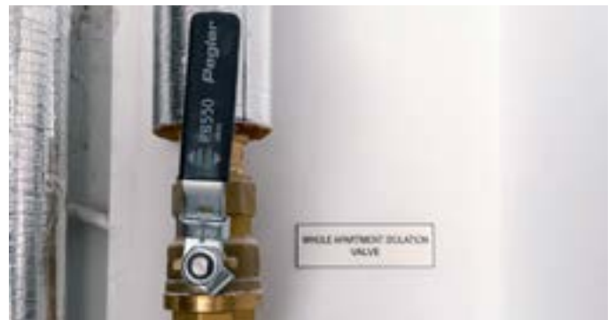
Stopcock inside utility cupboard
