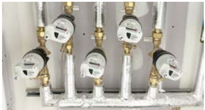
Stopcock in communal cupboard
