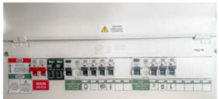
Indicative electrical consumer unit
