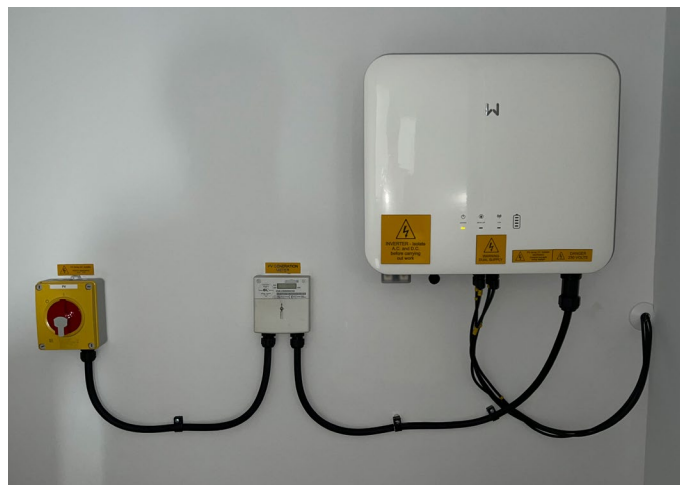
Indicative solar PV inverter
