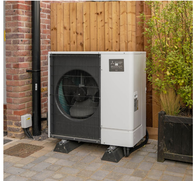
Indicative Air Source Heat Pump (ASHP)
